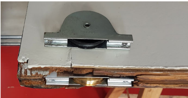
Fig. 9 Replacement of roller at the bottom of movable partition during repair works in 2019. Jurjen Creman.
